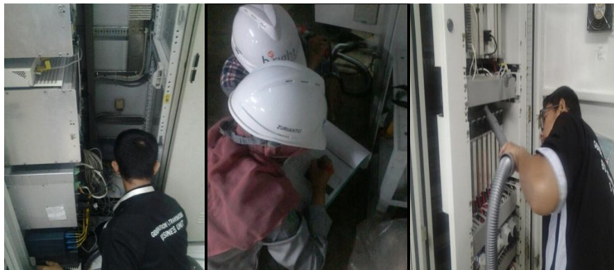
Gambar 18. Perawatan peralatan SCADA di remote station
