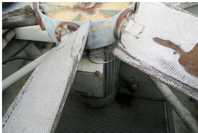
Gambar 3.5 charger air radiator fan a
