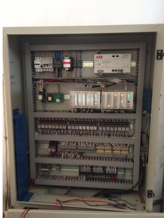
Gambar 25 RTU (Remote Terminal Unit)
